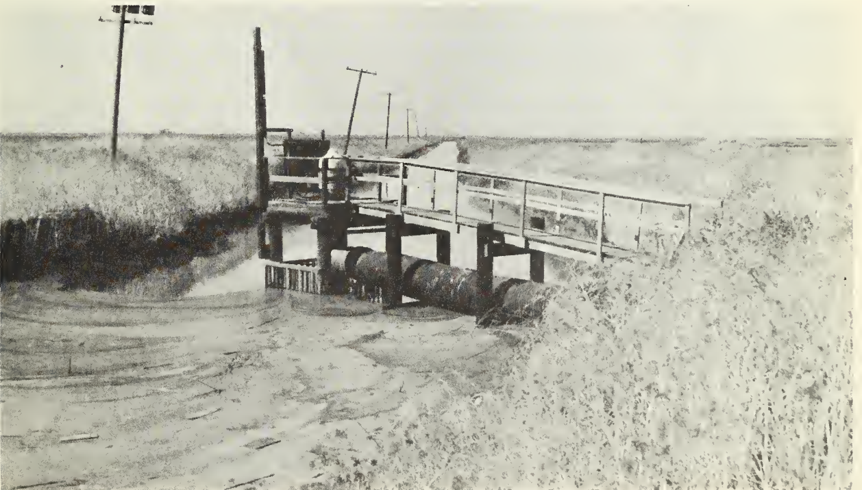
Photo 9. Pump installed for positive water control, independent of tides, particularly beneficial in draining.
